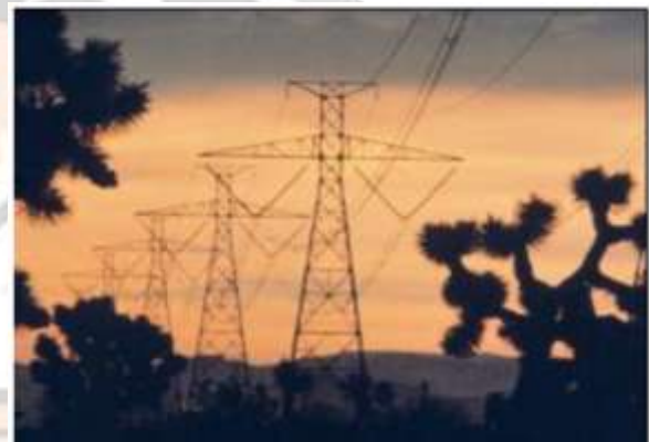
Fig. 2. \pm 500 kV HVDC transmission line
