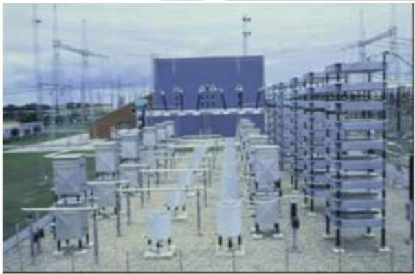
Fig. 1. HVDC converter station with AC filters in the foreground and valve hall in the background
