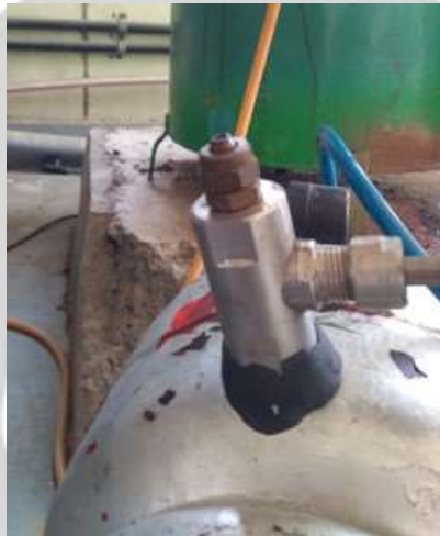
Fig. 4: Upgrade biogas flame
