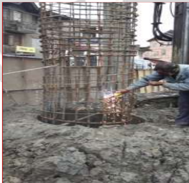
(3.2) Upper and lower cages are welded (using arc welding) to make it work as a single unit
