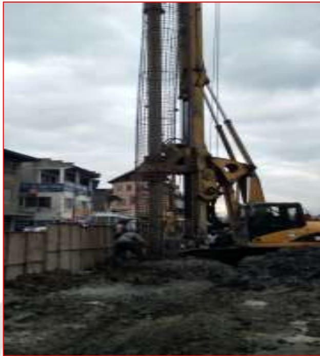
(3.1) Crane fitted within rig used to lift and drop reinforced cage into the pile bore
