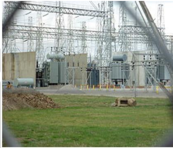
fig – 1 transformer at a power station
