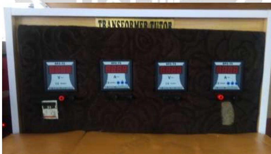
Figure4: Front view of the digital meters
