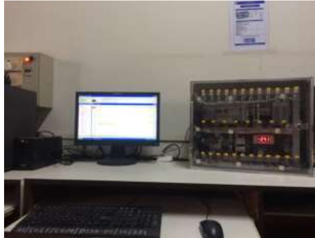
Fig -1: Allen Bradley PLC
