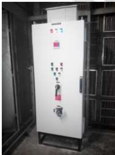
Fig-12 VFD Panel
