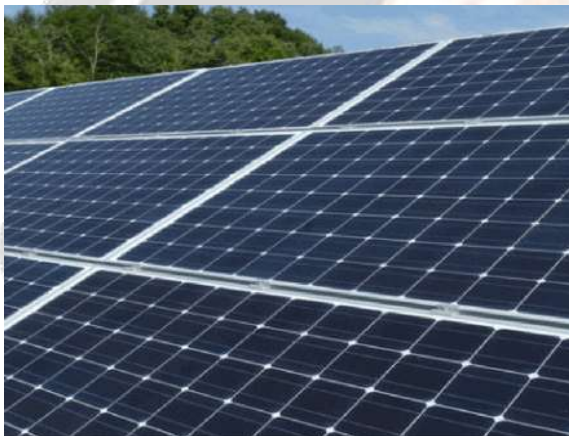
Fig :- Solar panel
