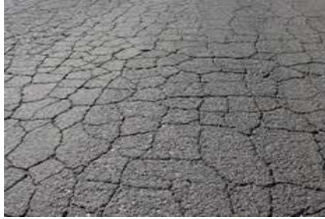
Figure 5: Failure in Rigid Pavement by Fatigue Cracking
