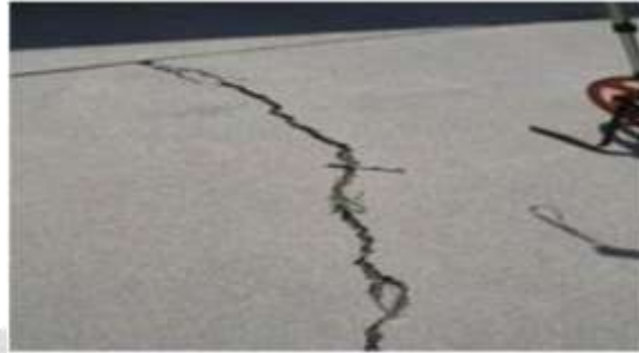
Figure 1: Failure in Rigid Pavement by Linear / Longitudinal Cracking
