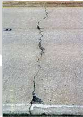
Figure 2: Failure in Rigid Pavement by Transverse Cracking
