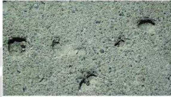
Figure 10: Failure in Rigid Pavement by Pop out
