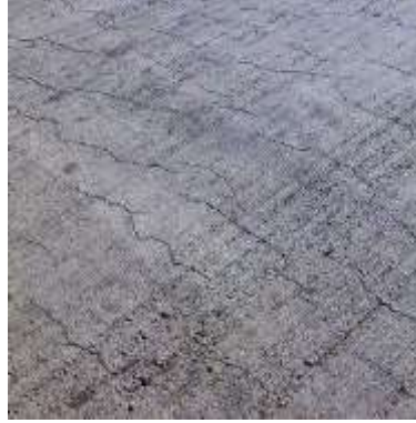
Figure 3: Failure in Rigid Pavement by Shrinkage cracks
