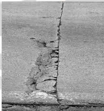
Figure 12: Failure in Rigid Pavement by Spalling
