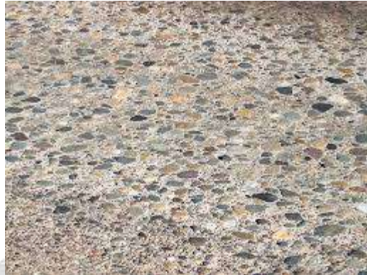
Figure 12: Failure in Rigid Pavement by Aggregates with polished surfaces
