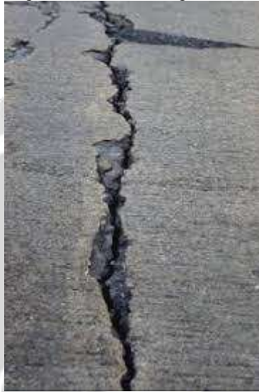
Figure 8: Failure in Rigid Pavement by Faulting
