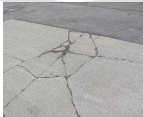
Figure 7: Failure in Rigid Pavement by Punch Out
