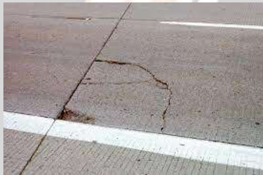
Figure 6: Failure in Rigid Pavement by Corner Break Cracking
