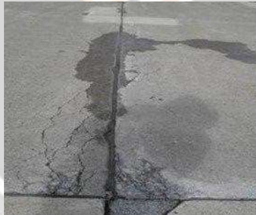
Figure 4: Failure in Rigid Pavement by Durability Crack
