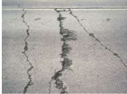
Figure 11: Failure in Rigid Pavement by Pumping
