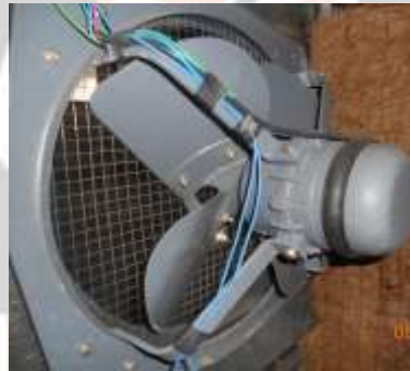
Figure no: 3.1 Fan
