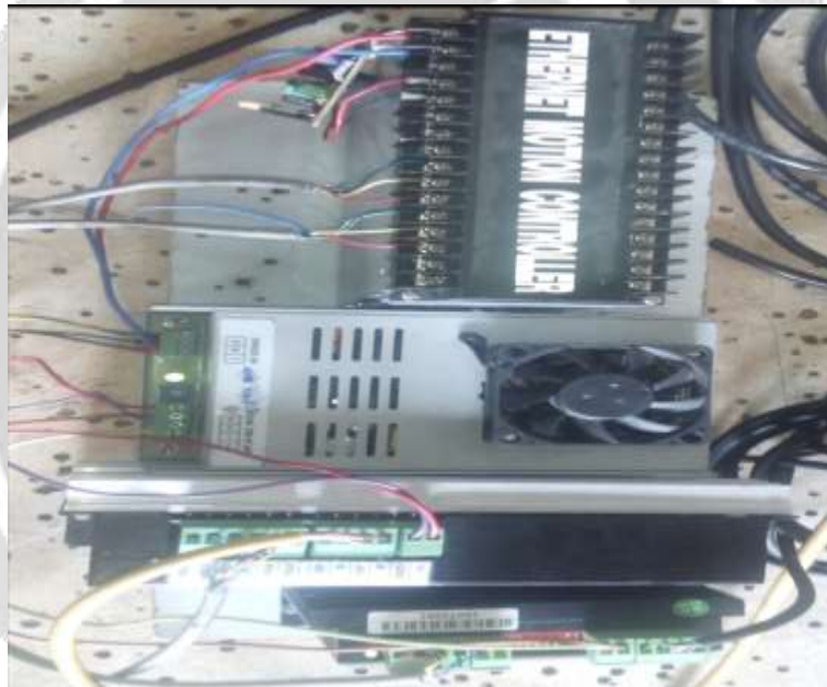
Fig- 5: Electrical Control Panel
