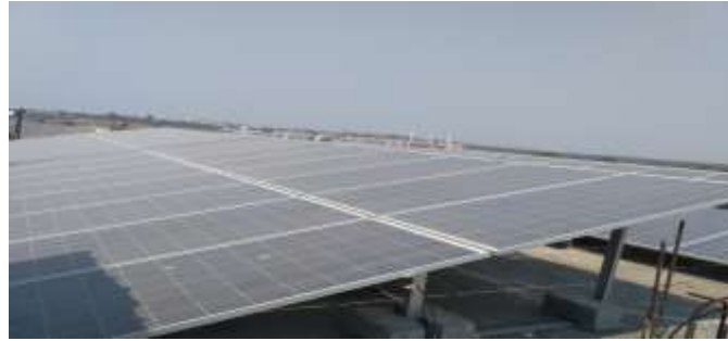
Fig .3 Actual onsite of 30KW solar roof top plant at St.Peter's International School, Hyderabad City
