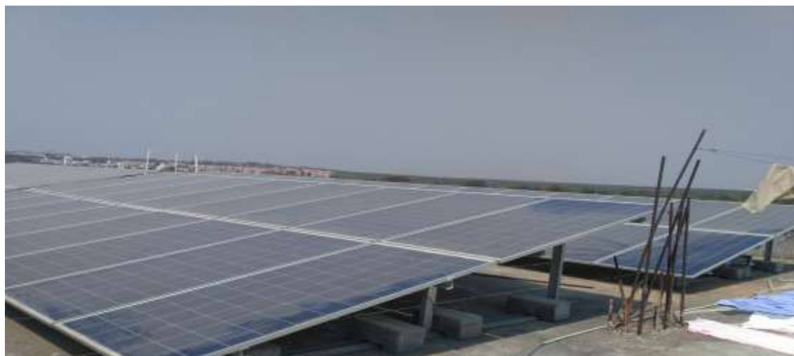
Fig.4 Actual onsite of 30KW solar roof top PV modules at St.Peter's International School, Hyderabad City
