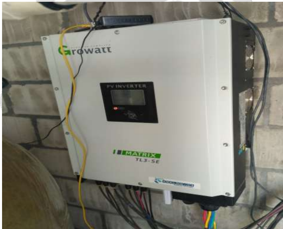
Fig.5 Actual onsite 30KVA solar grid inverter at St. International School, Hyderabad City
