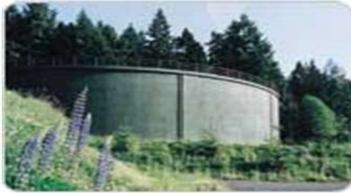
Fig 1.2: Ground water tank
