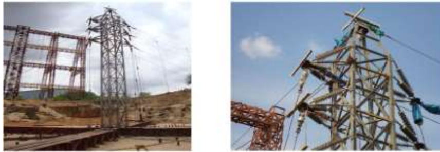
Fig.1. Rigging arrangement of composite tower Fig.2 Calibrated load cells attached to the on the tower test bed composite cross arm
