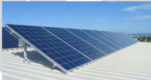
Fig. 3.1.1 Solar Panel (A)
