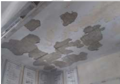
Fig 1- spalling of paint
