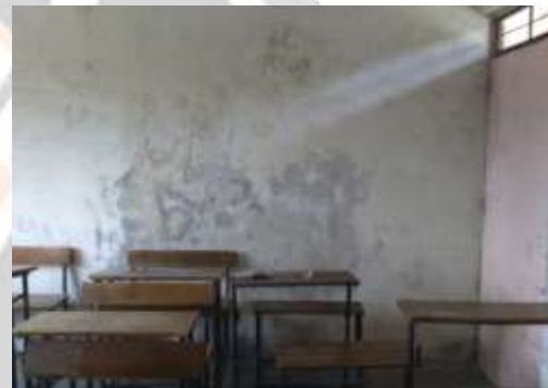
Fig 2- seepage of water through walls
