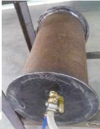
Fig-3 Air Tank
