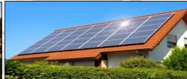
Fig -8: PV Roof [47]
