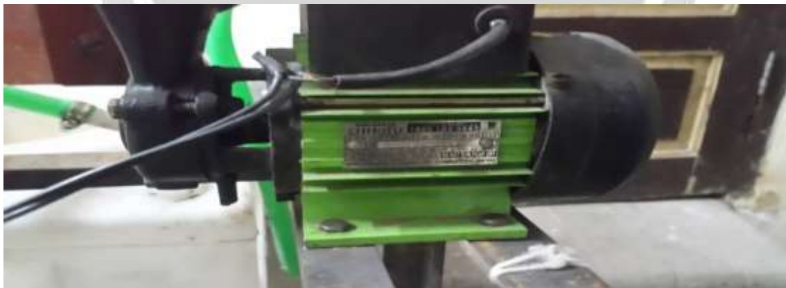
Figure 3.3 Pump and motor for operating Machine
