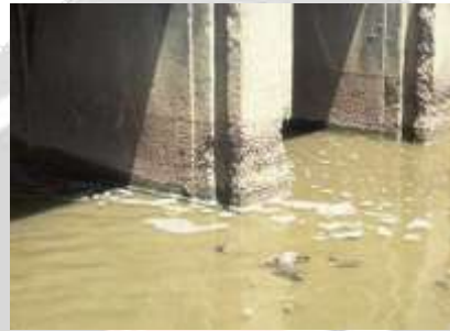
Fig 1.1: Photograph of bridge pier corroded by acid water.
