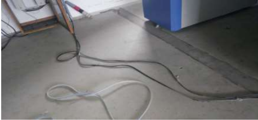
Fig -2:Exposed Electrical Parts
