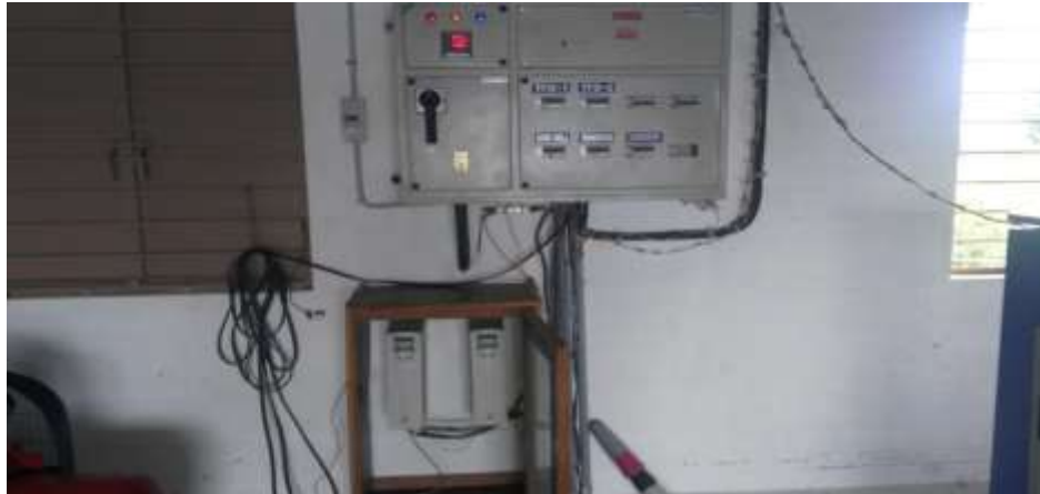
Fig -3:Unsafe Work
