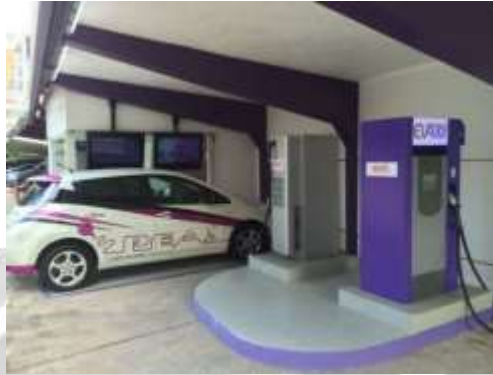
Fig. 1 Quick charging station for EVs.
