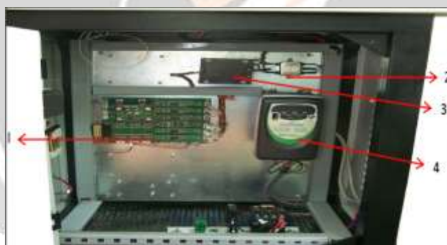
[1] I-DAS card [2] line filter [3] transformer [4] AC drive
