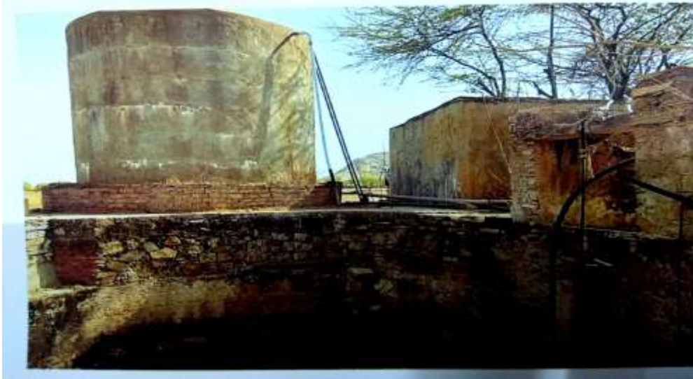
Dry Well Akhri Village
