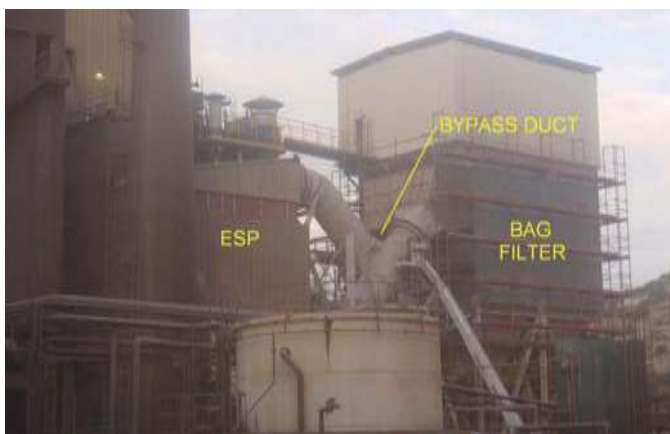
Figure 1: Example of a hybrid dedusting system constituted by an ESP coupled with a bag filter.
