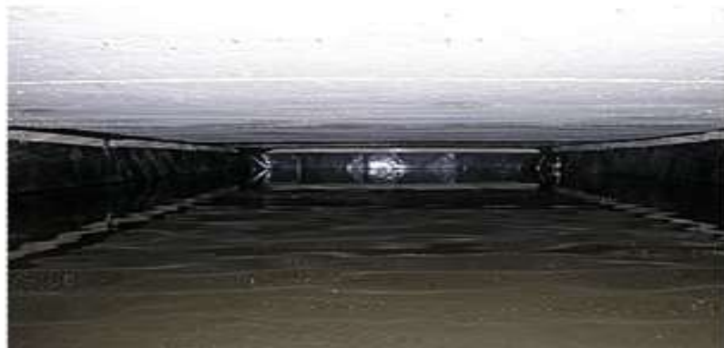
Fig 1.2.2: Underground water tank
