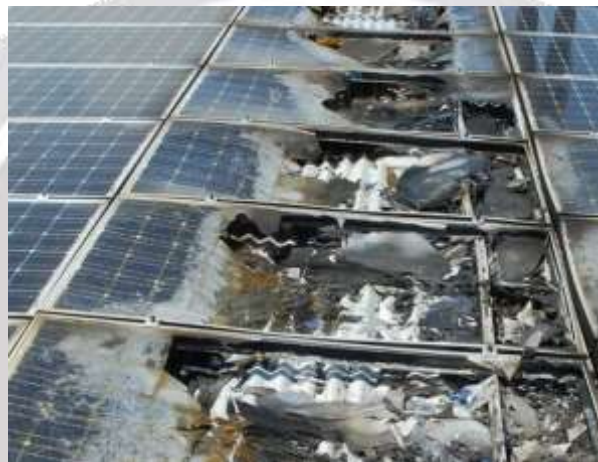
Fig 1.1 (b) fault occurred in 1 MW PV power plant in Mount Holly, North Carolina, in 2011
