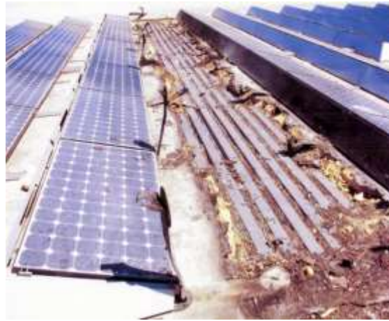
Fig 1.1(a) fire hazard in a 383 kW PV array in Bakersfield, California in 2009
