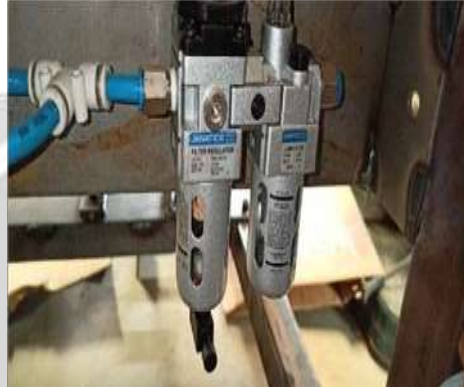
Fig-3 valves with air control system.
