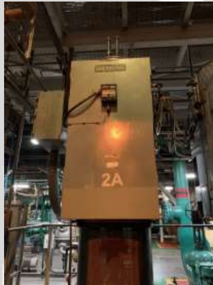
Fig -1 Motor Condensate Pump 2A (CP)
