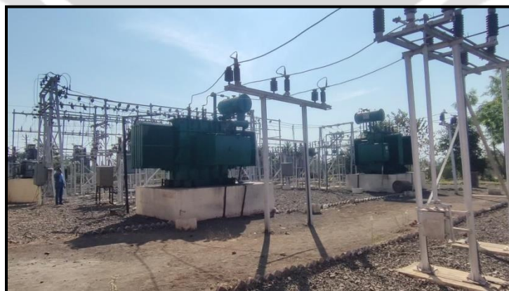
Fig -1 : 33/11 kV Substation
