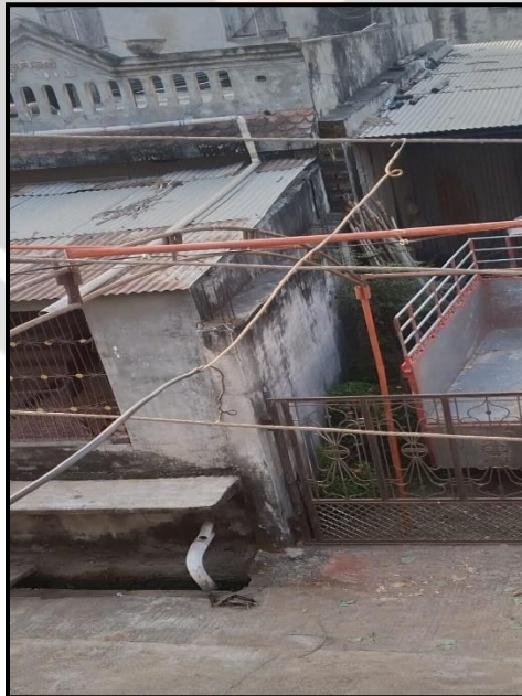
Fig -2 : Illegal Hooking
