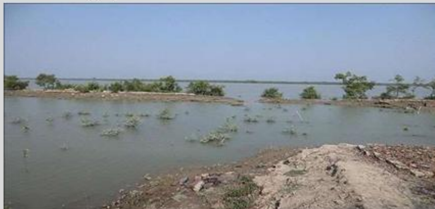
Plate 1 The broken embankment by the storm surge of SCS, Aila in 2009
