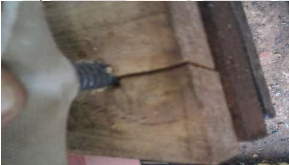
Figure 4.2.4: Crack Prorogated near Discontinuity of Wood Plank
