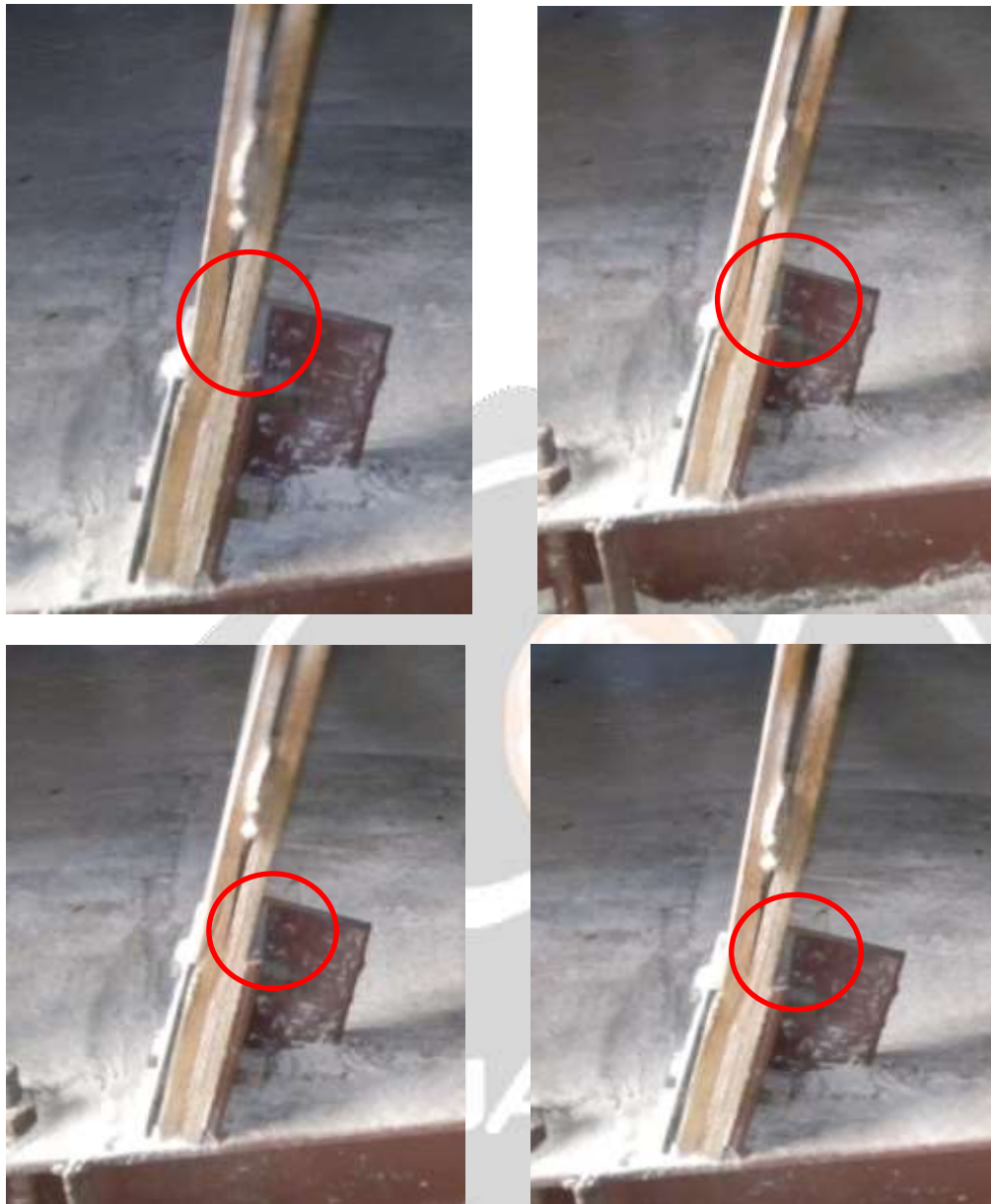
Figure 4.3.1: Failure of Wooden Plank
