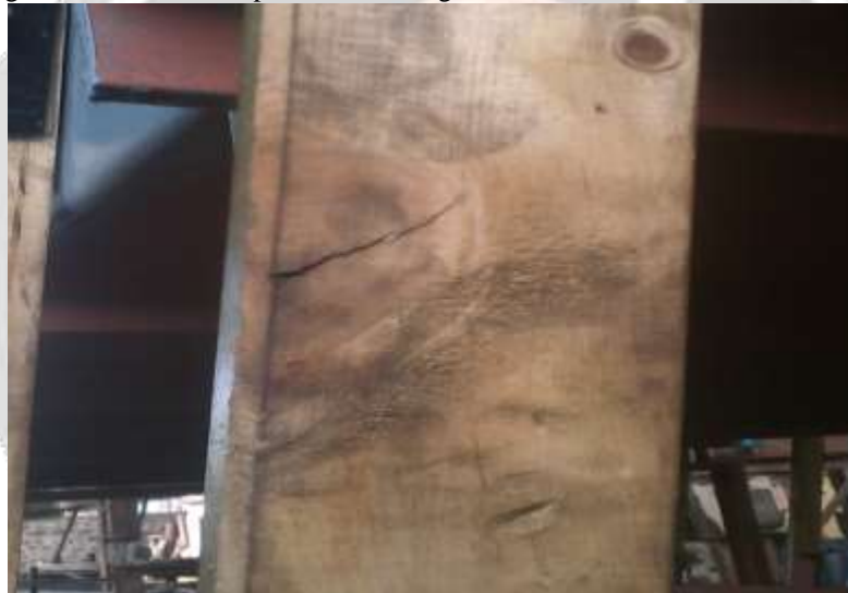
Figure 4.2.2: Failure Cause by Tension in Wooden Flank Assembly
