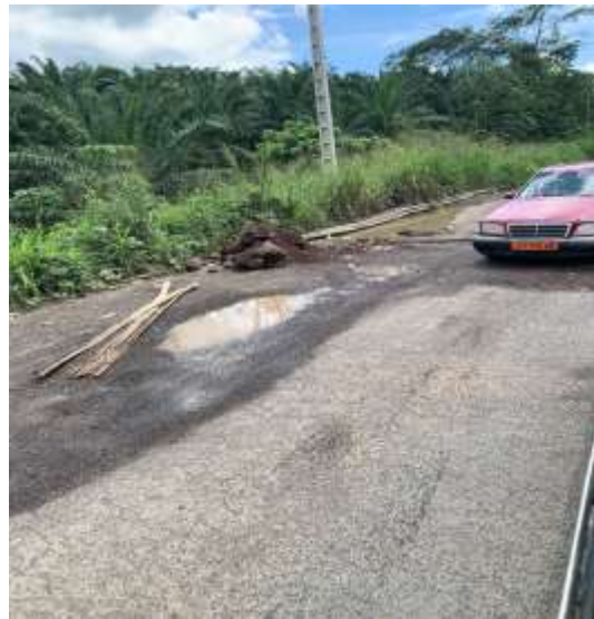
Figure 3. Rut and depression with worn out guardrails extending to the road lane at Mbanga entrance
