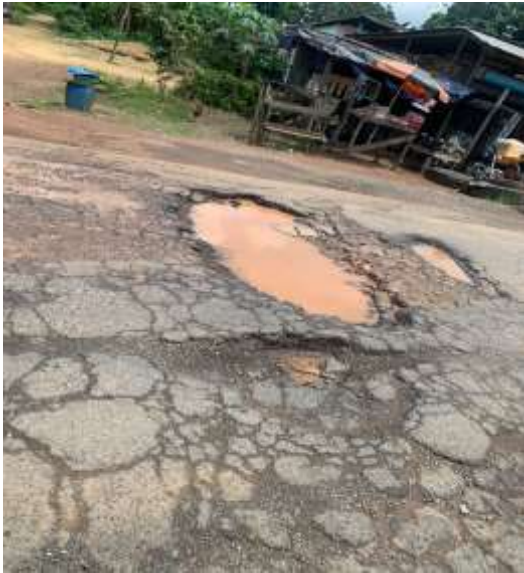
Figure 2. Delaminated and cracked road filled with potholes at Bomono
