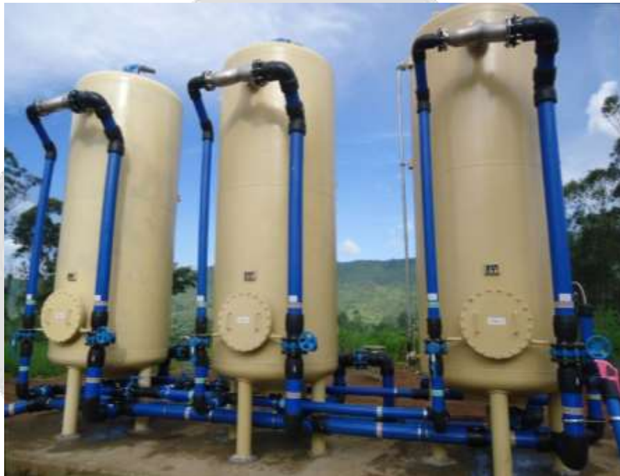
Picture 1: Bamenda III Water Purification Plant
