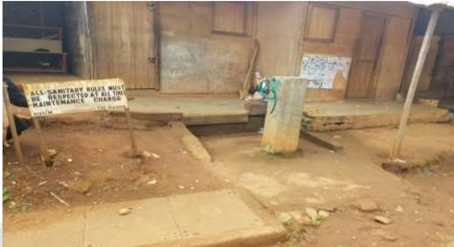
Picture 3: Abandoned stand tap at Foncha Street, Bamenda III Municipality.
