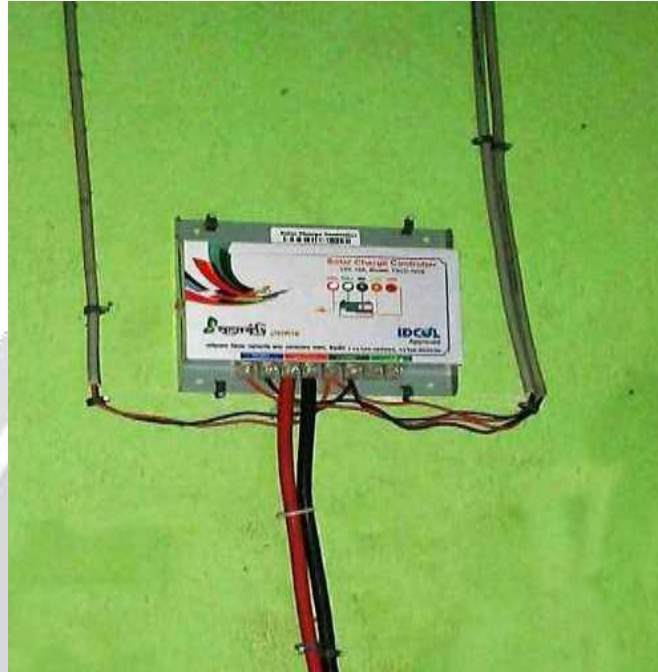
Figure 2- 5: Pico-Solar Charge Controller Setup in the House wall
