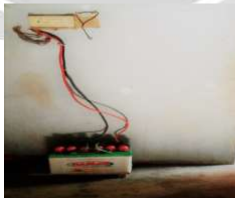
Figure 2- 6: Rechargeable Battery setup in the house of SHS
