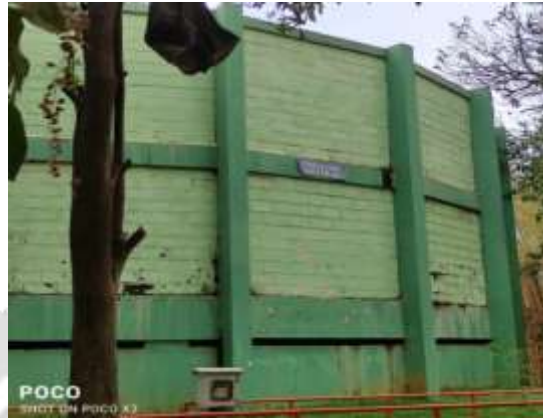
Fig6: Vrishabhavathi Valley Wastewater Treatment Plant trickling Filter.
