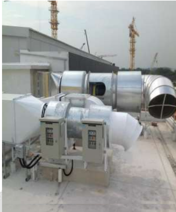
Fig: Exhaust air outlet in Industries
