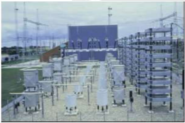
Fig. 1. HVDC converter station with AC filters in the foreground and valve hall in the background
