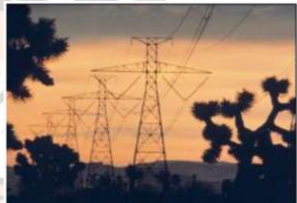
Fig. 2. \pm 500 kV HVDC transmission line
