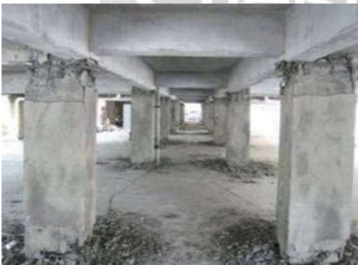
Fig. 1: Columns in the bottom open story of a six-story building, after undergoing plastic hinge due to the earthquake
