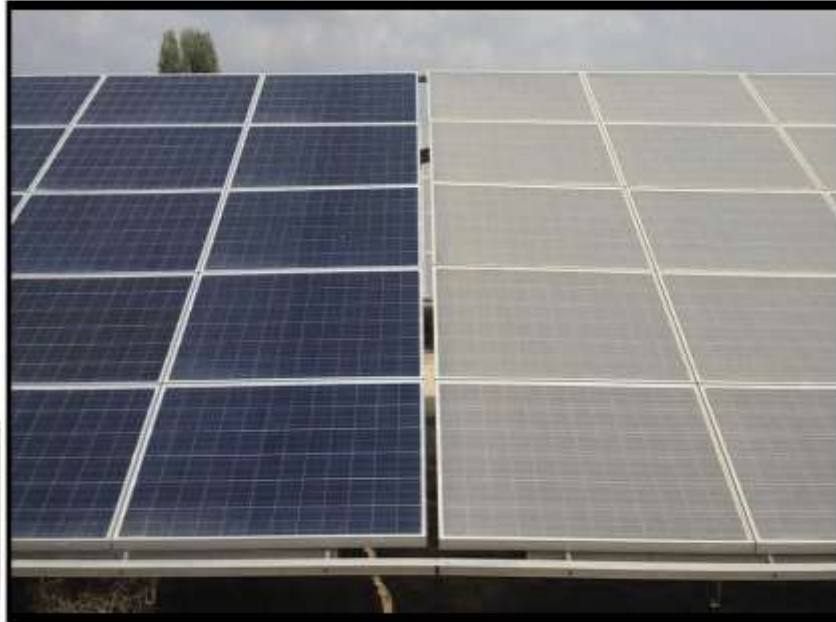
Fig.1 Solar module covered by heavy layer due to dust accumulation before cleaning
