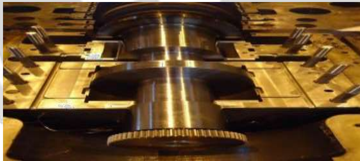
Fig 2. Turbine base plate with front bearing pedestal
