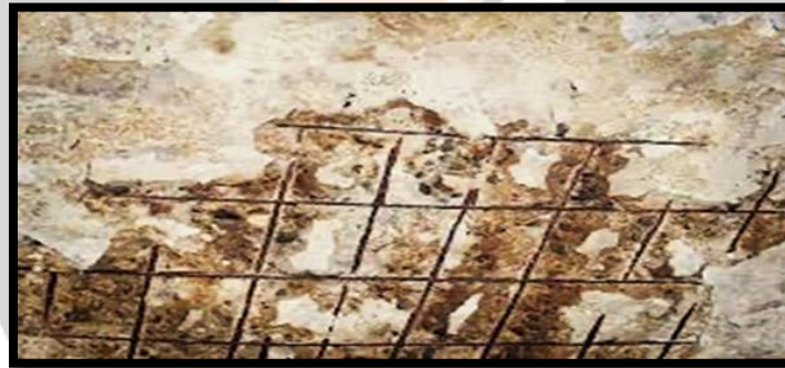
Figure. 2 Reinforcement corrosion on water tank
