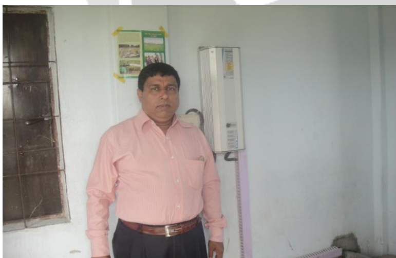
Fig.3 A control room for maintaining the liaison among solar panel, water pump and loads.
