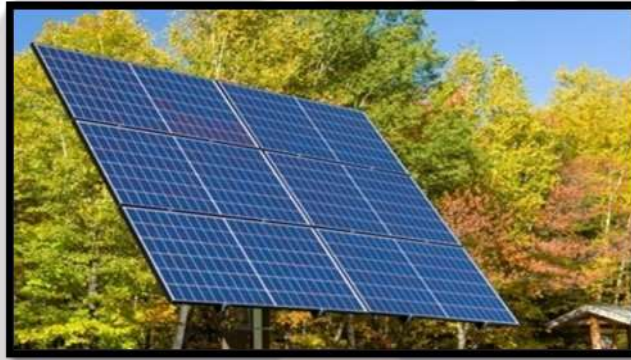
Fig -3: Solar Panel
