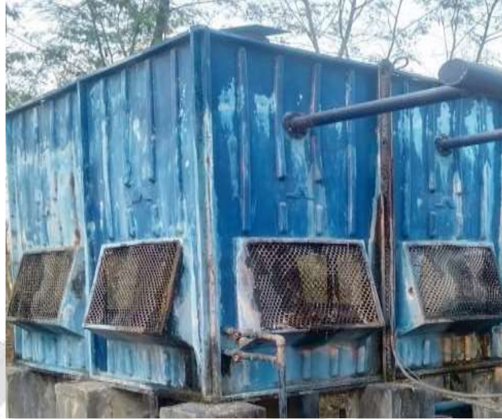
Fig. 3: Practical of Cooling Tower
