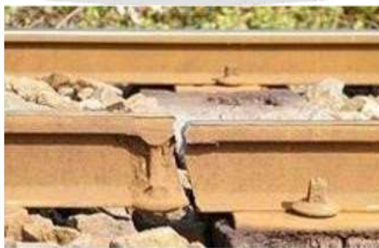
Fig.1. Railway crack on track
